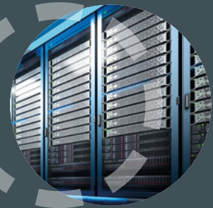
Fig 1c: Optical interconnects enable high-speed communication between processors in a data center.
